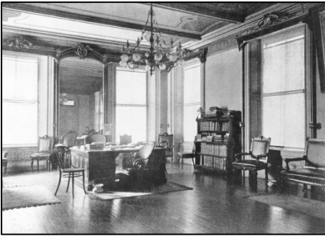
This original ceiling in Room 3316 is now hidden behind another decorative ceiling.
